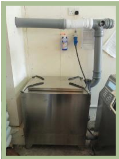
The bio filter unit with outlet pipe
